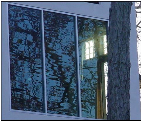
Figure 1: Example of optical distortion viewed in reflection from a glass surface
